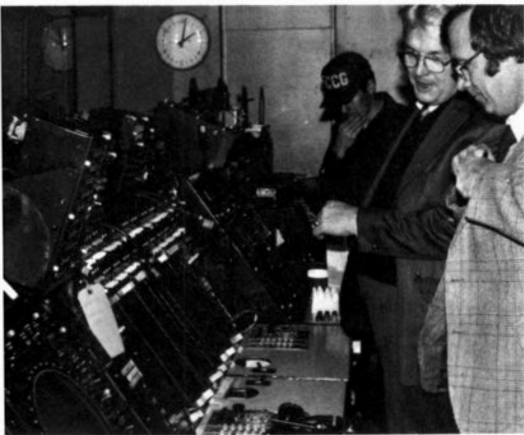
Charles Weaver of the region's Airway Facilities' Communications Staff discusses the trailer-borne TRACON with a telephone company representative.
